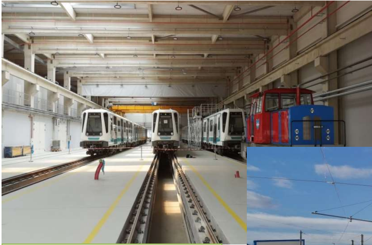
General view and working halls in the constructed metro depot of Line 3
