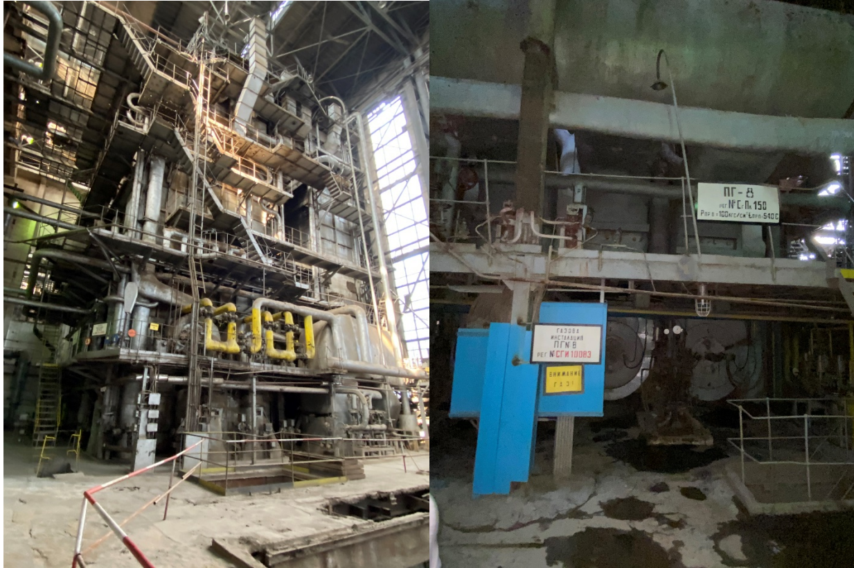
Figure 2-1 Site Visit Pictures of Some Boilers
